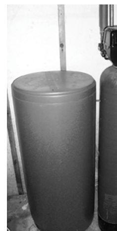
Above: Water Softener
