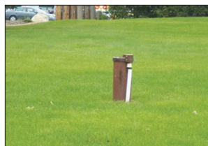
Photo above: well with broken electrical conduit.
